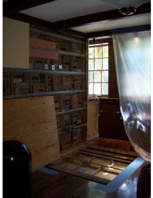
Photo #2: Floor and wall opened exposed
