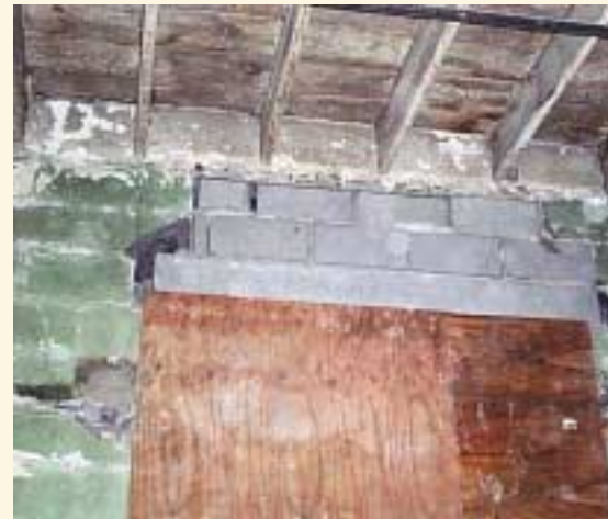
The existing masonry dividing walls were in very poor condition.
