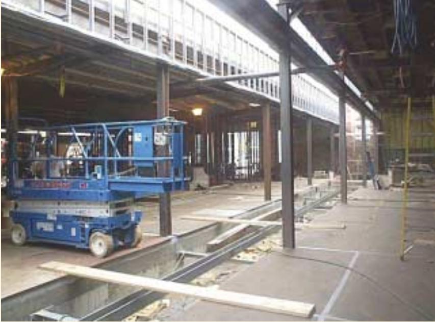
CMU walls dividing each building from an enclosed alley were replaced with new steel framing. The old alleys (the narrow area between the columns in this picture) became atriums.
