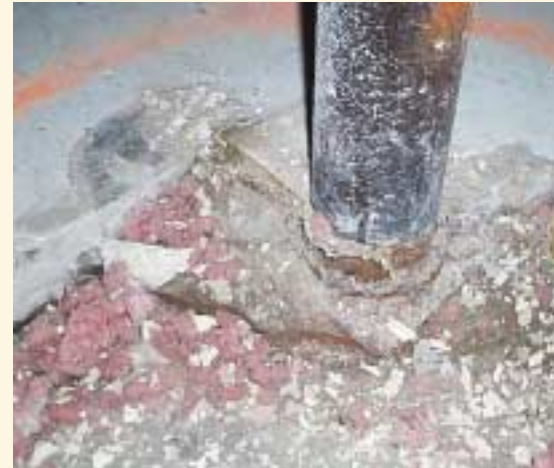
Many existing column bases were deteriorated.
