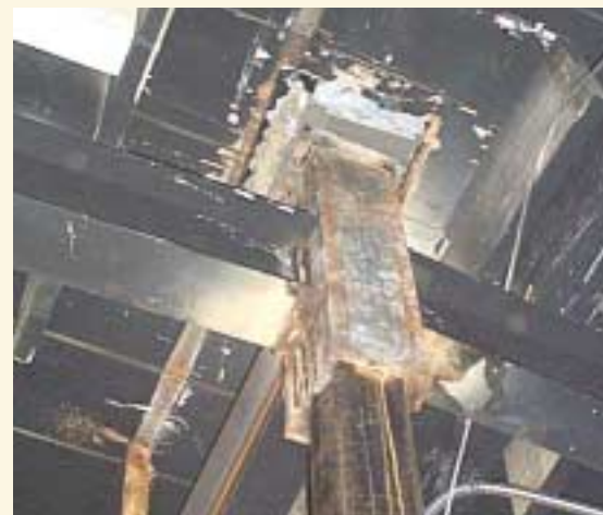
Channels attached to each side of the existing columns extend through the roof to support additional loads.
